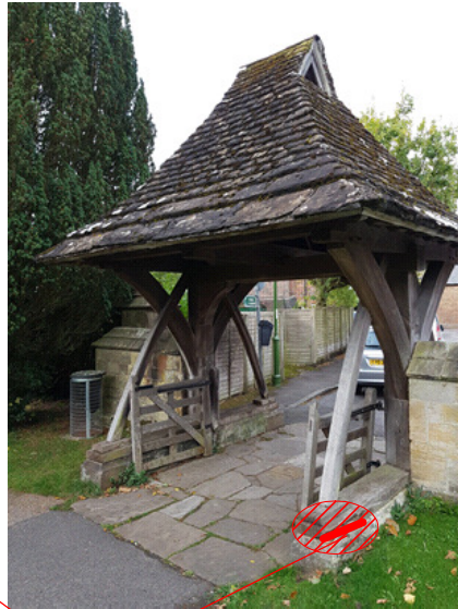
Decay and insect damage to the underside of the sole-plate on the Church side of the gate
