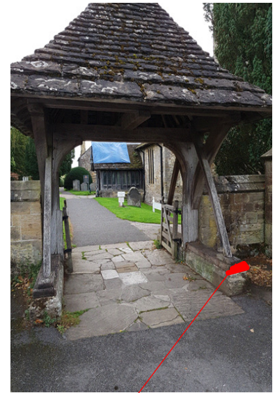
Decay and degradation at the outer end of the sole-plate on the outer side of the gate
