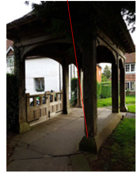
Some decay evident in the base of the rear right corner vertical support
