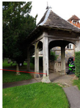
Rear left corner post showing long vertical crack in the timber support
