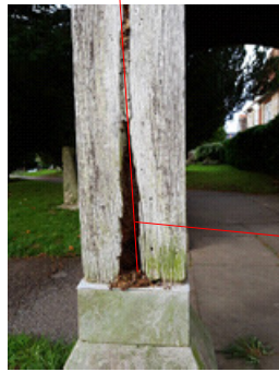
Decay and insect damage to base of vertical support, plus large vertical crack in the timber
