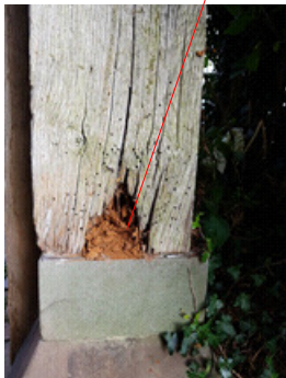
Decay and insect damage to base of vertical support. There is also a vertical crack on the outside, L/H side
